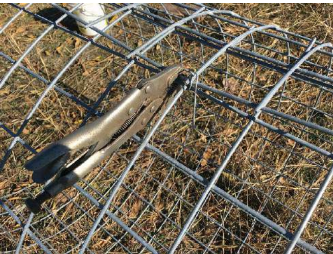
Fig 7.6: Using vice grip locking pliers to hold mesh together on a steel guard so tie wire can be fastened.
