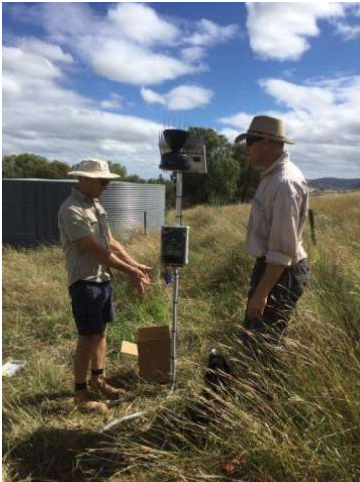
Paul Hudson from Cropsol Consulting Services with HCLG Chair Gordon Refshauge during installation of one of the soil moisture probes
